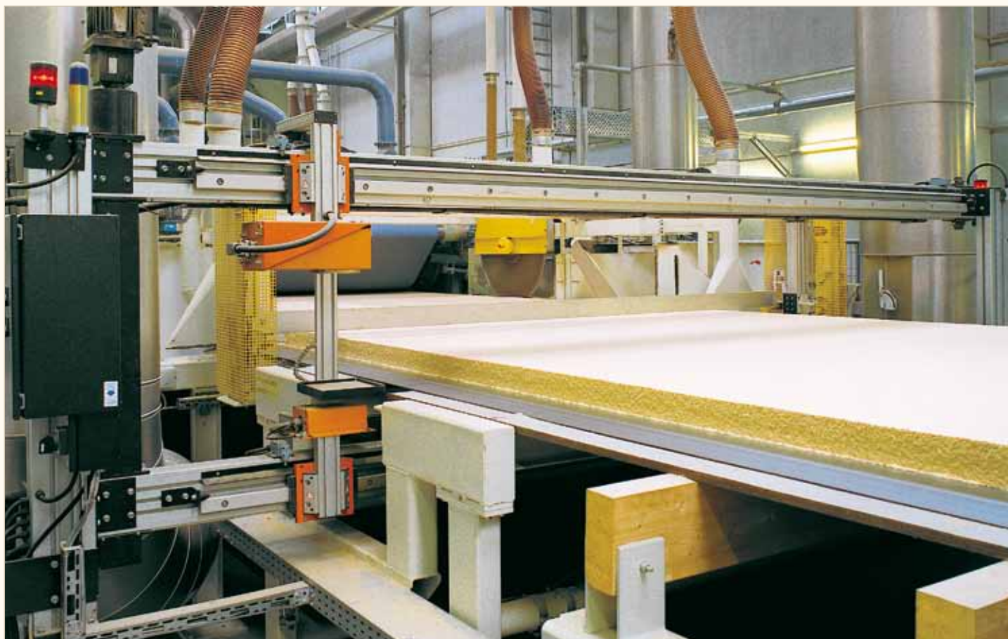
Measurement transducer in the calibration position
